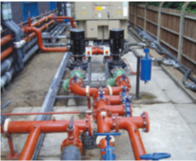
With the bulk of the new pipework installed, the entire system relied on the flexible hosing by the fence to the right feeding temporary chillers set up on site.
