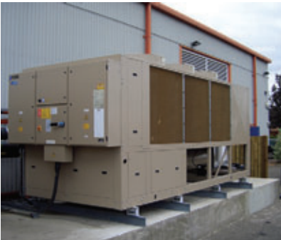
One of three high efficiency screw compressor chillers utilising ozone friendly Hfc R134a refrigerants and featuring fully modulating stepless control
