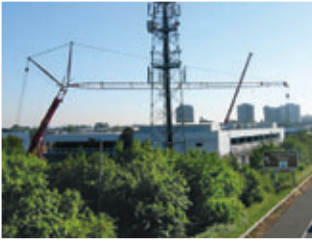
300 tonne mobile crane with maximum extension jib to span across the building
